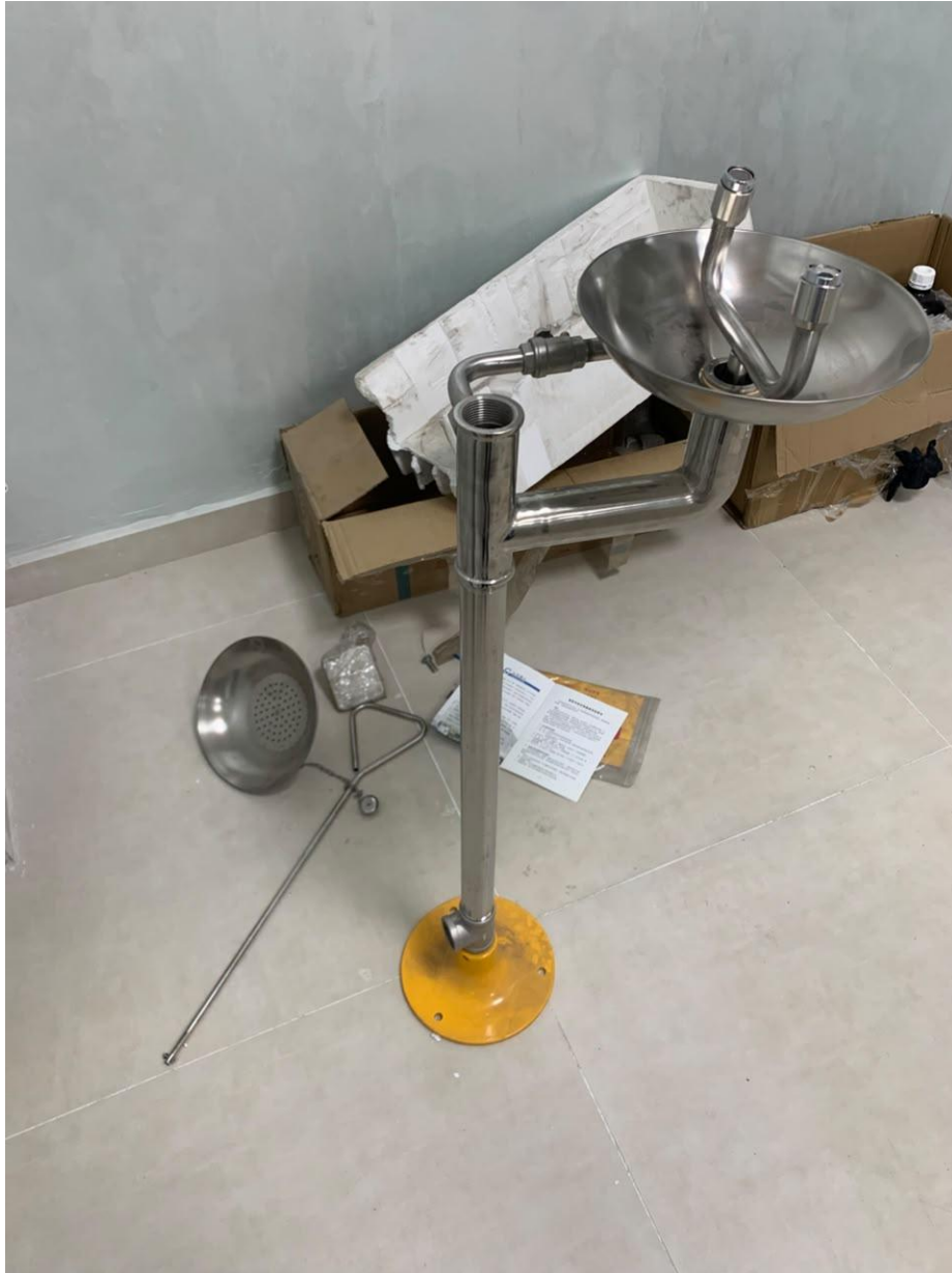
Figure 9.6: Stainless steel Emergency Eyewash and Safety Shower Unit installed for chemical splash decontamination.
