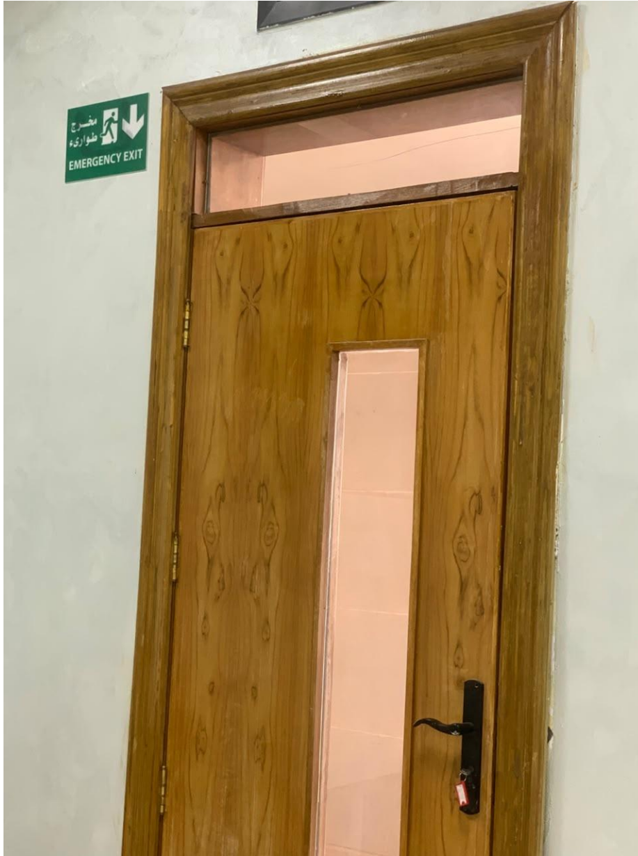
Figure 9.7: Emergency Exit door equipped with illuminated exit sign and panic opening hardware.
