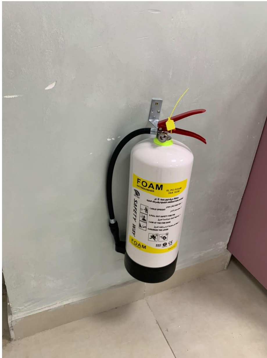
Figure 9.8: Wall-mounted 6L Foam Fire Extinguisher positioned near chemical processing areas.
